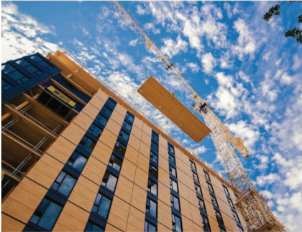
Work on the 18-storey Brock Commons building in Vancouver. The project was seen as a major step forward for mass timber.
