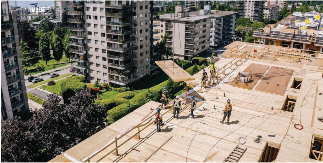
PHOTO: ADERA A CLT panel being hoisted into place on Adera's Crest project.
